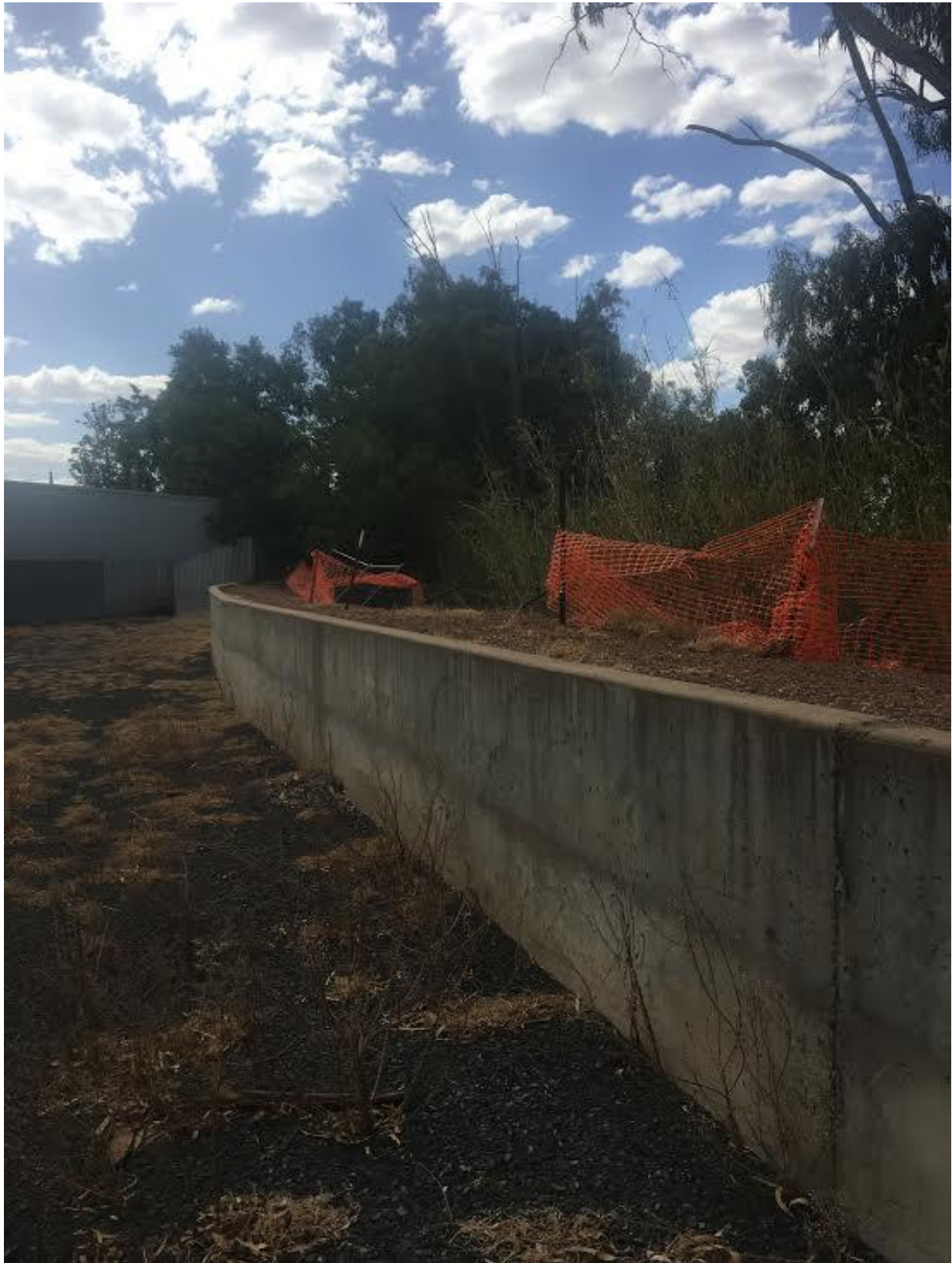
Photograph 13 Dentist Surgery/Courthouse Retaining Wall
