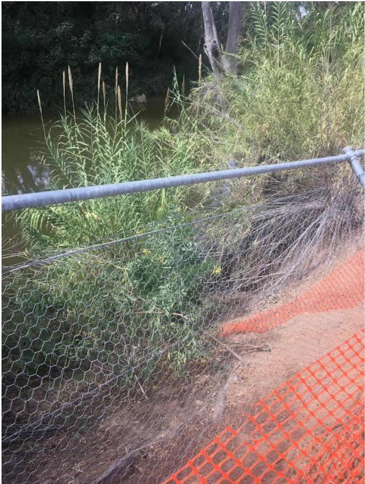
Photograph 7 Dentist Surgery/Courthouse Slippage
