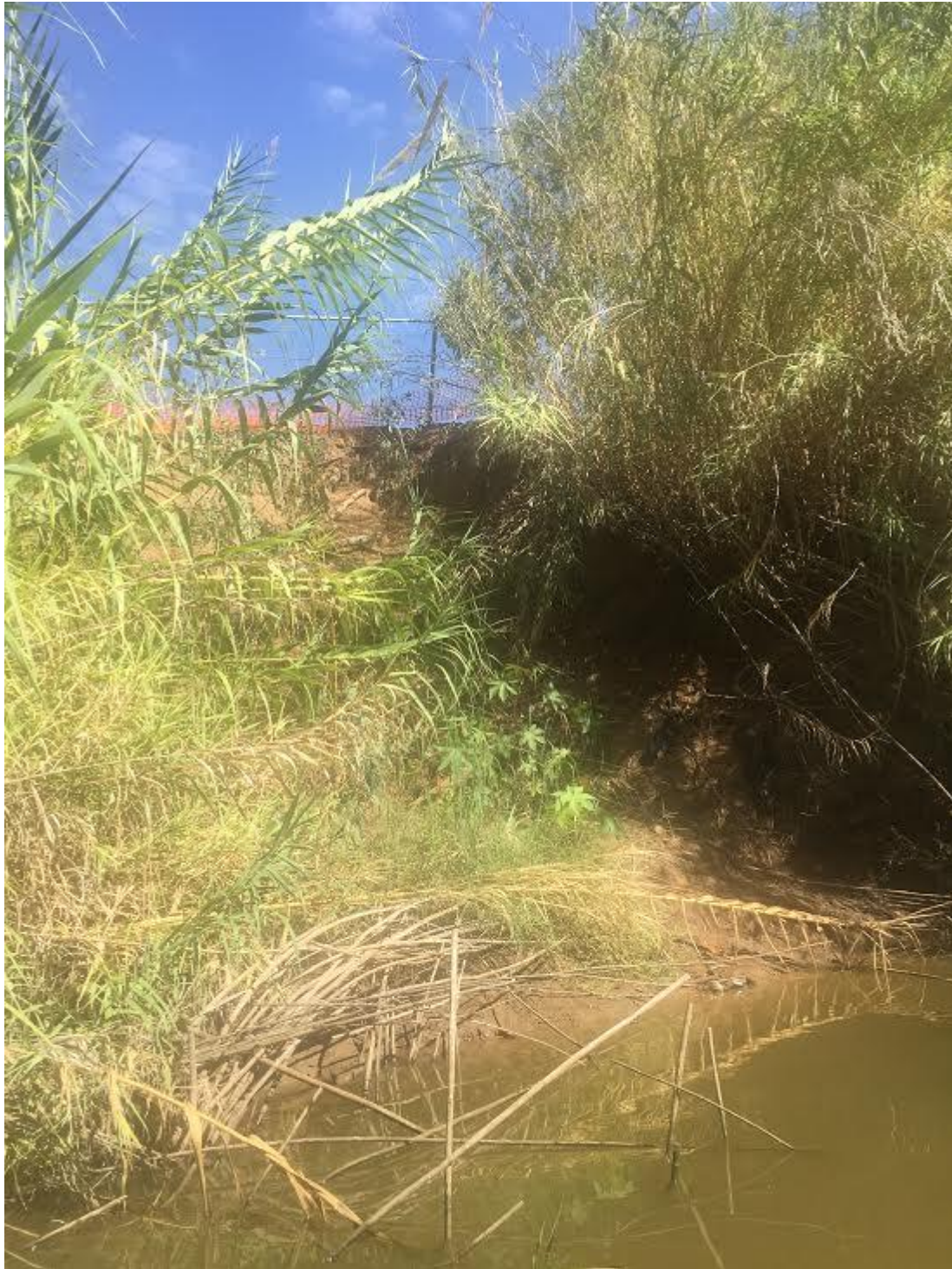
Photograph 3 Dentist Surgery/Courthouse Slippage
