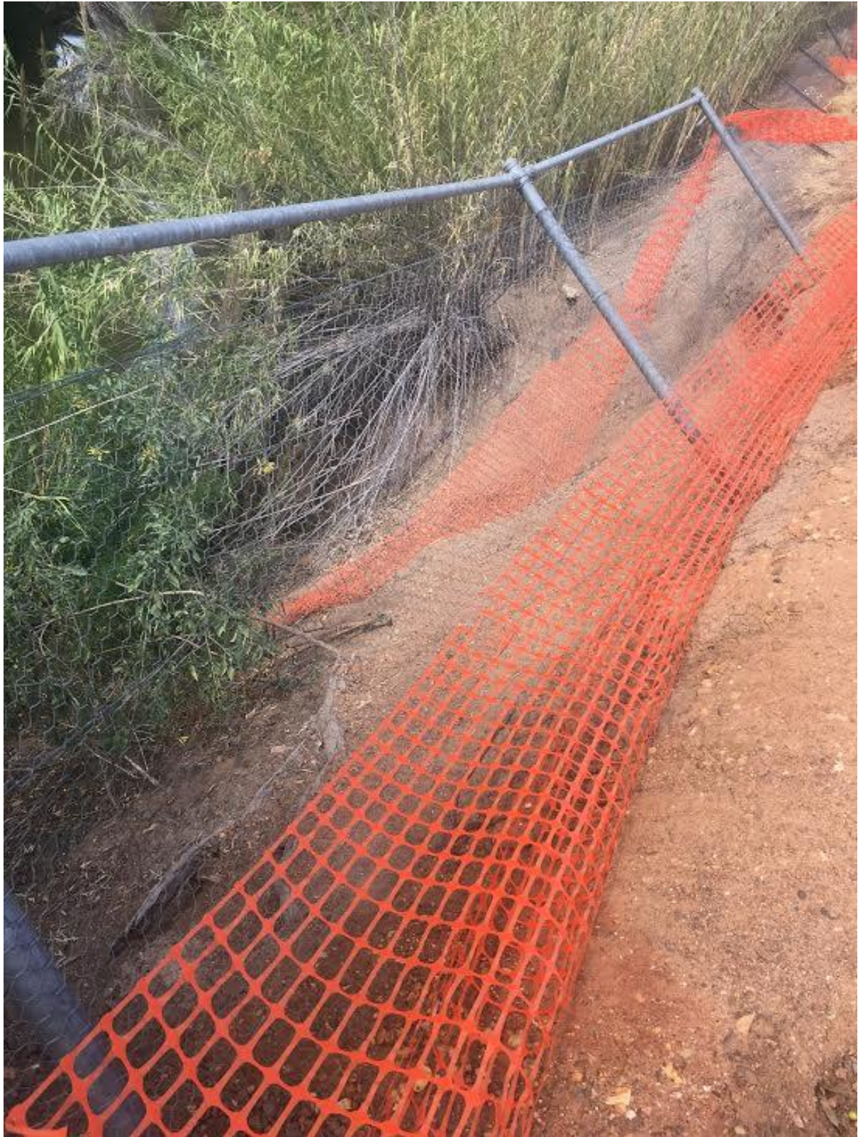
Photograph 6 Dentist Surgery/Courthouse Slippage
