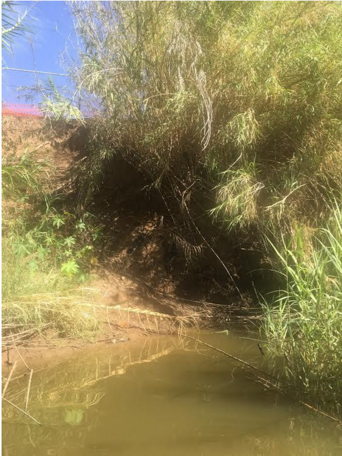
Photograph 2 Dentist Surgery/Courthouse Slippage
