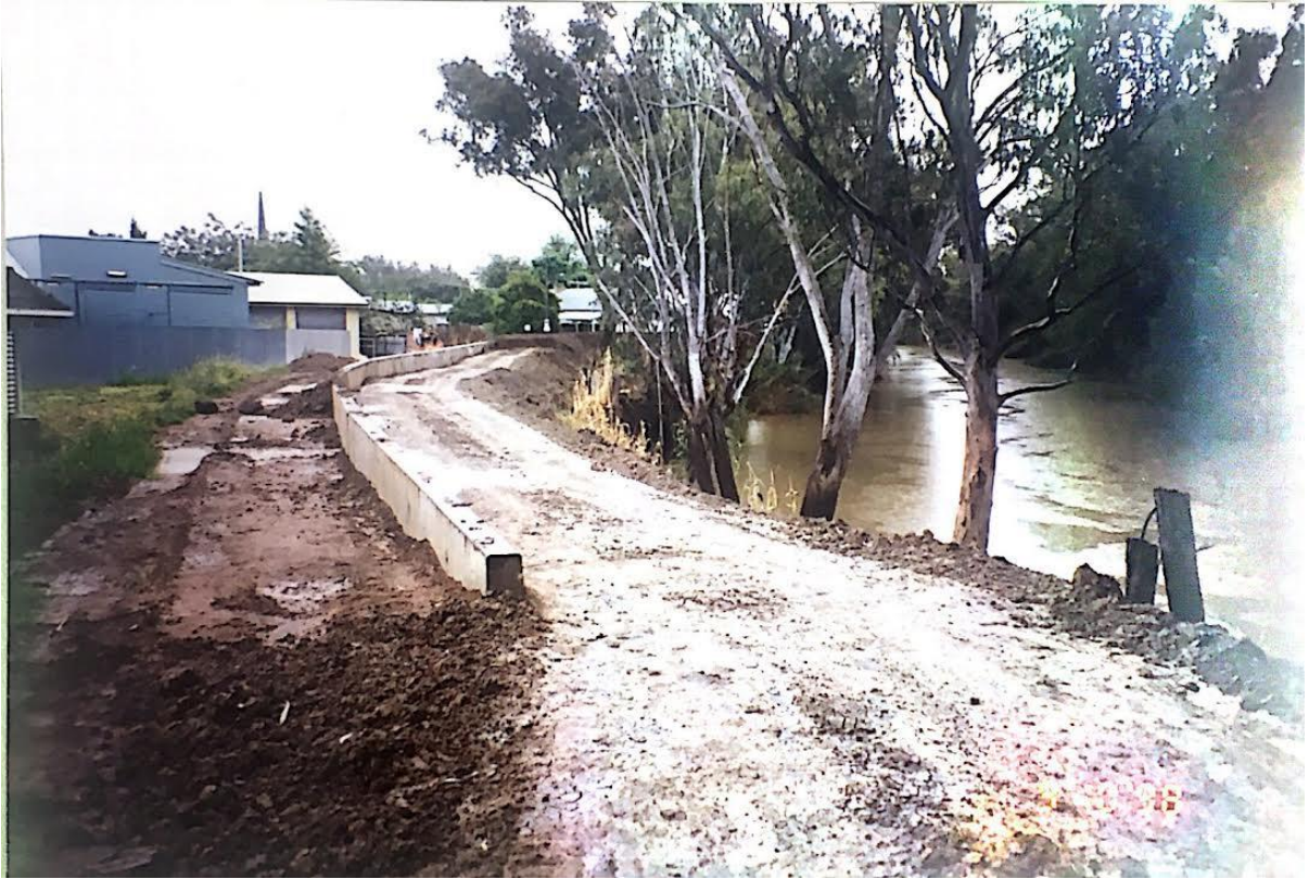
Photograph 20 Dentist Surgery/Courthouse Retaining Wall
